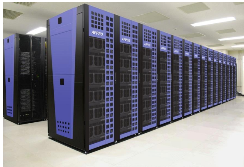
Figure 138. A cluster organized in cooled racks
